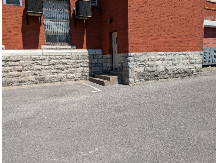
Picture 1: Picture taken from the back of building toward the Exist. Exit from the building is not level to the ground level.
